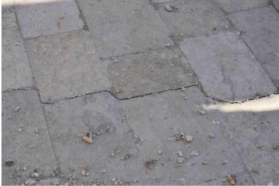
Cracks and cracks in the floor of the Ottoman bath in Manbij
