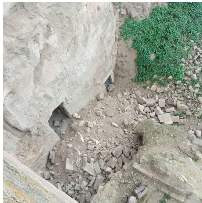
Structure collapse in Najm Castle
