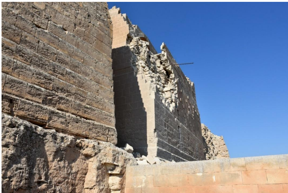
Parts of the outer wall of Najm Castle collapsed near the main entrance
