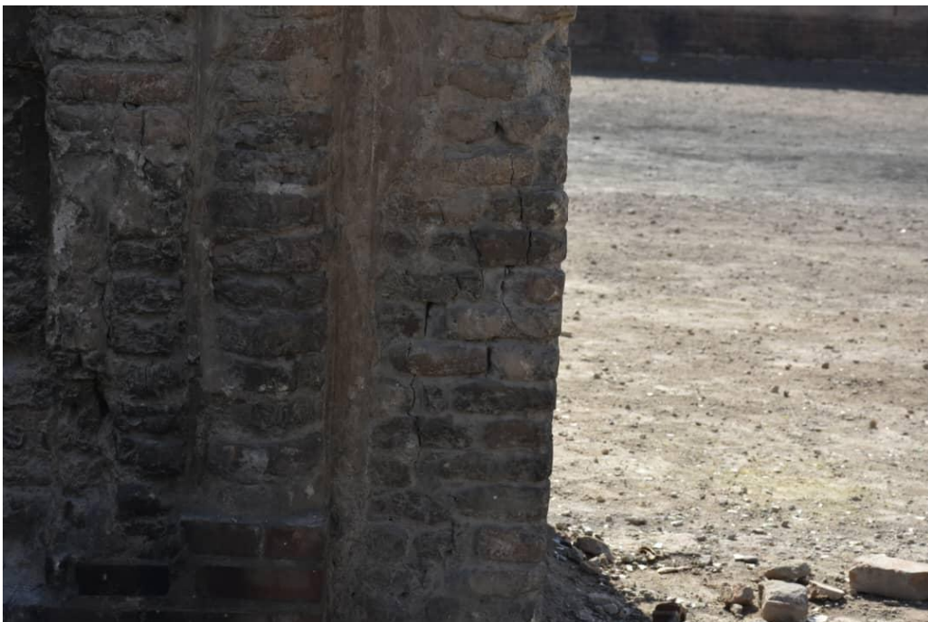
Minor cracks in the arched walls of the ancient mosque in Raqqa.
