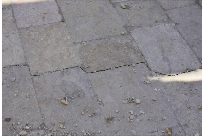
Cracks and cracks in the floor of the Manbij Citadel Mosque
