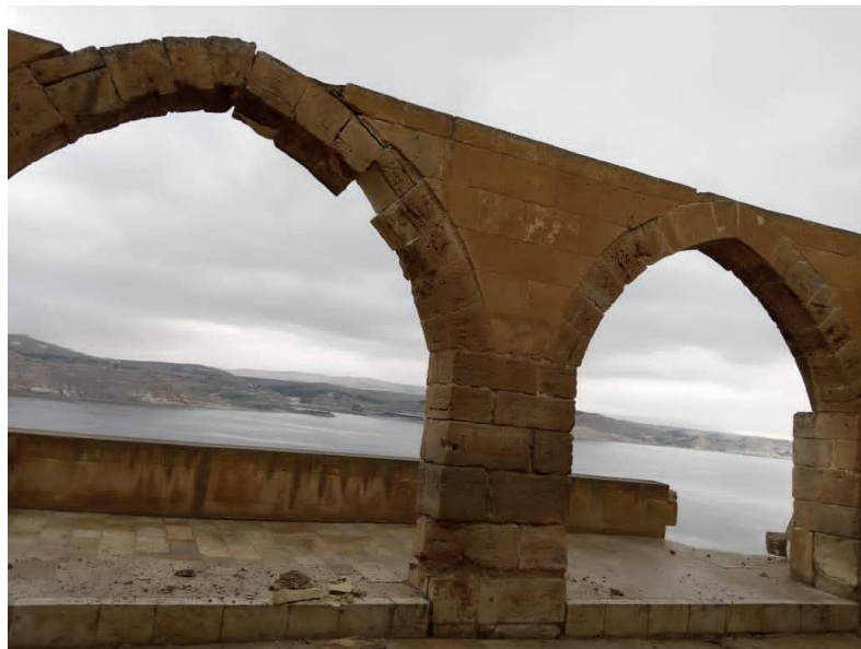
New cracks in the arches of Najm Castle
