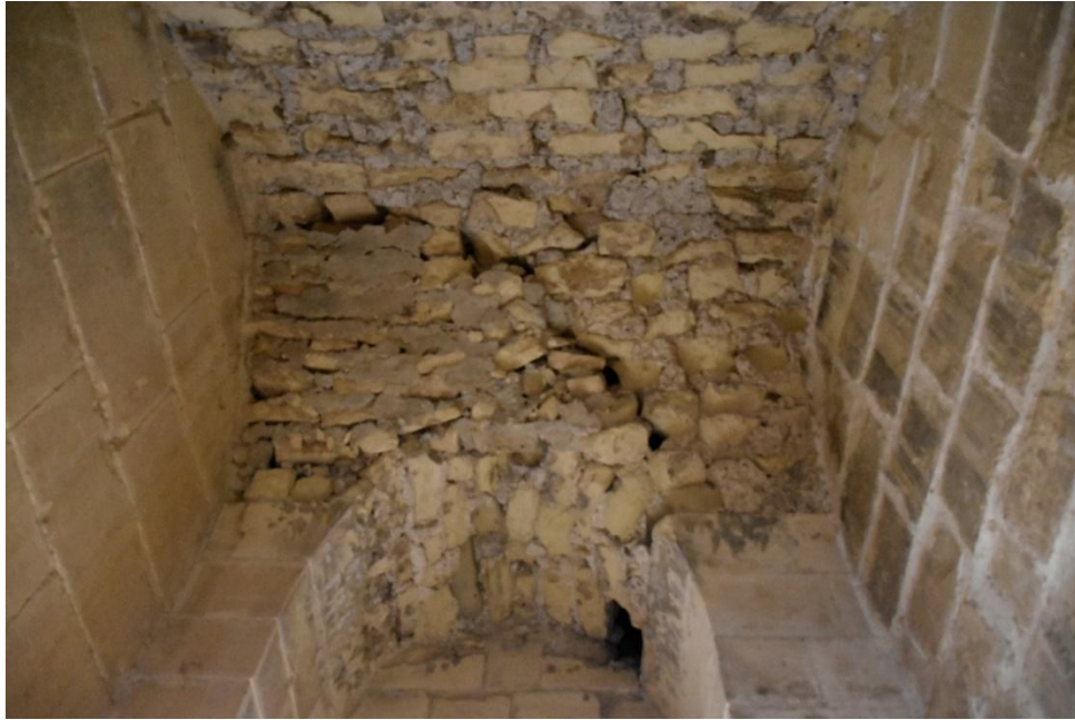
Cracks in the ceilings of the throne room at Najm Castle
