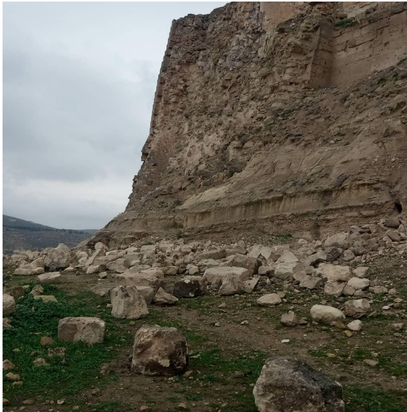
Collapsed parts of the outer wall of Najm Castle
