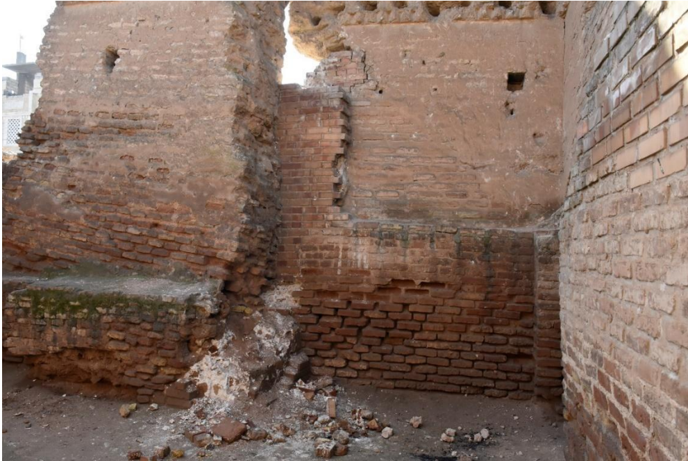
A slight crack and collapse of parts of one of the walls in the Banat or Girl's Palace in Raqqa
