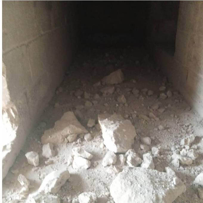
Structure collapse in Najm Castle
