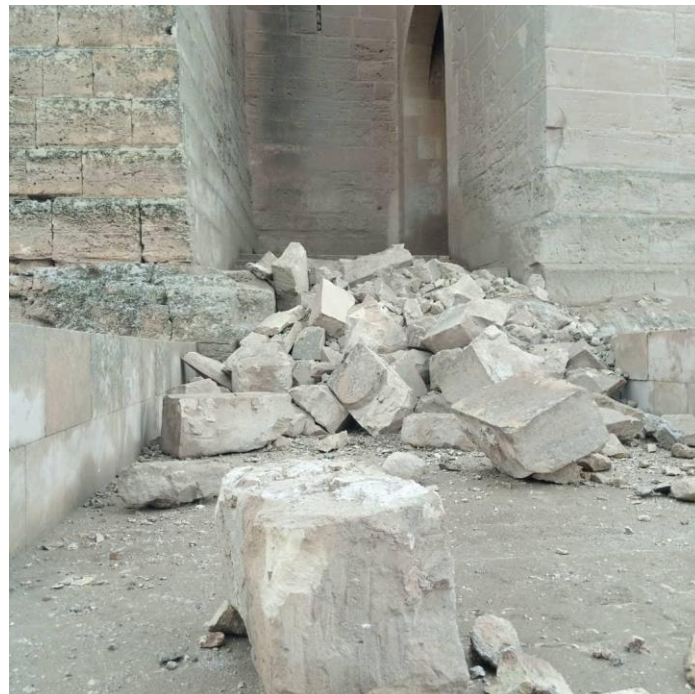
Structure collapse in Najm Castle
