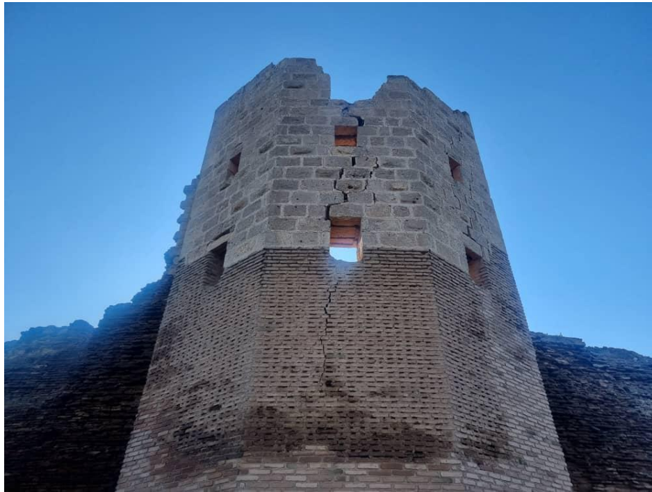
Cracking in the Gharib Tower at Ja'bar Castle
