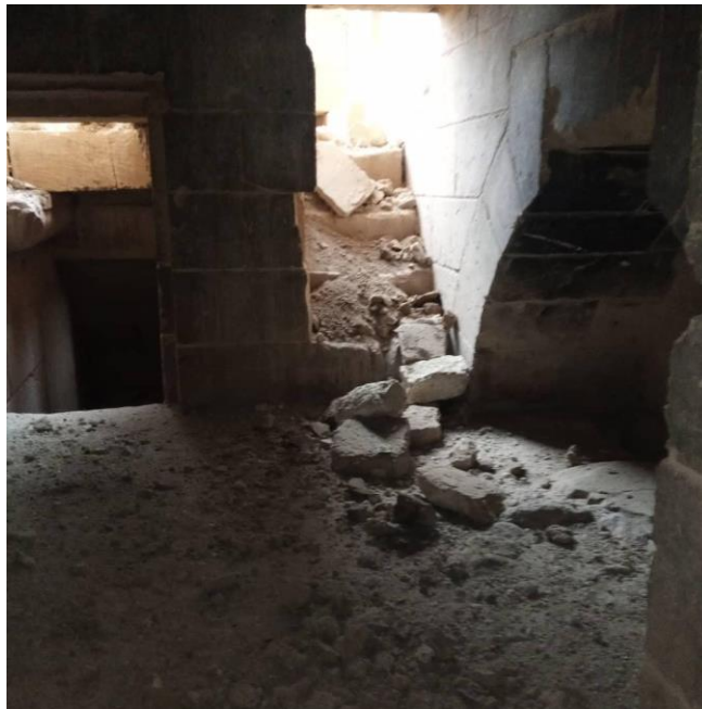
Structure collapse in Najm Castle
