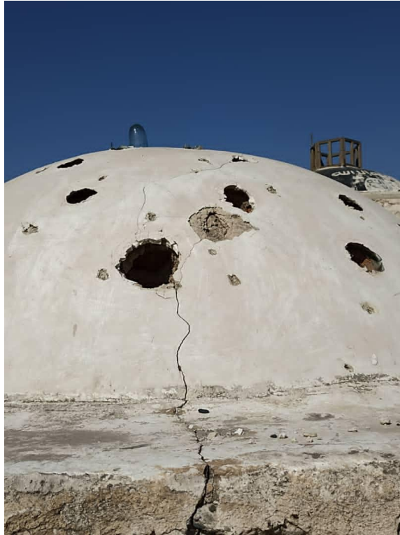
Cracks in one of the domes of the Ottoman bath in Manbij
