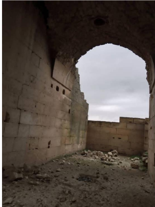
New cracks and fractions in the arches of Najm Castle
