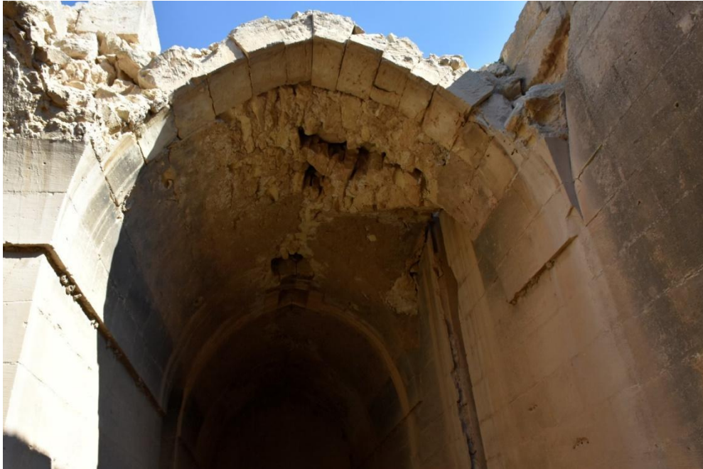
Cracking and collapsing of some stones from the roof of the court in Najm Castle
