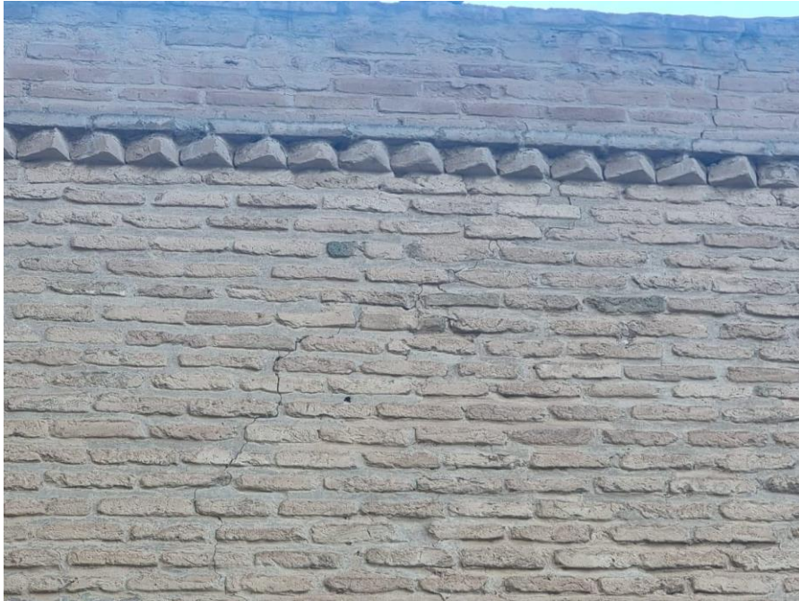
A crack in the outer façade of Alia Tower (the façade of Jaabar Castle Museum)
