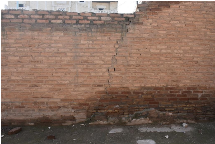
A crack in one of the walls of the Girls' Palace in Raqqa
