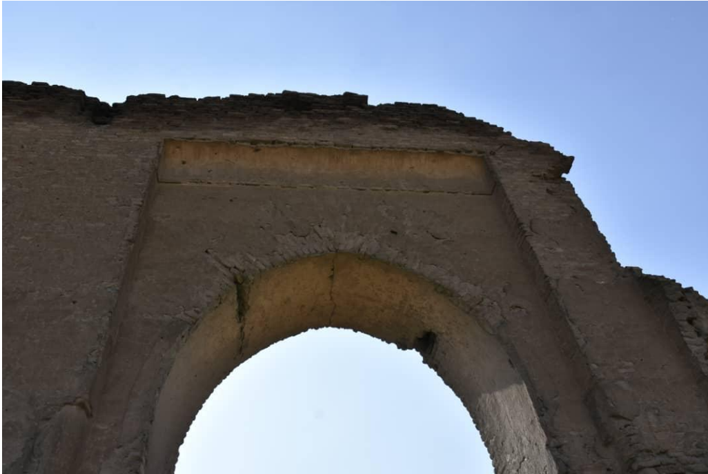
Cracks in one of the arches of the ancient mosque in Raqqa
