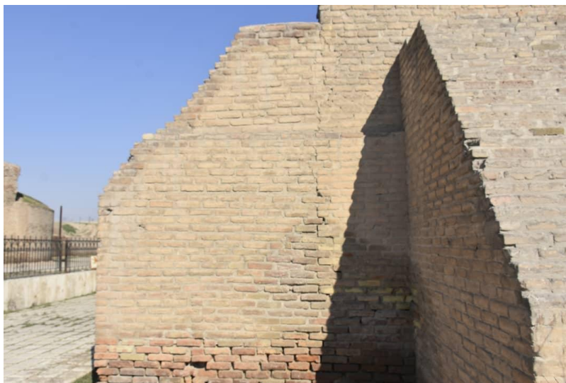
The crack on the other side of the pillar supporting the Baghdad Gate
