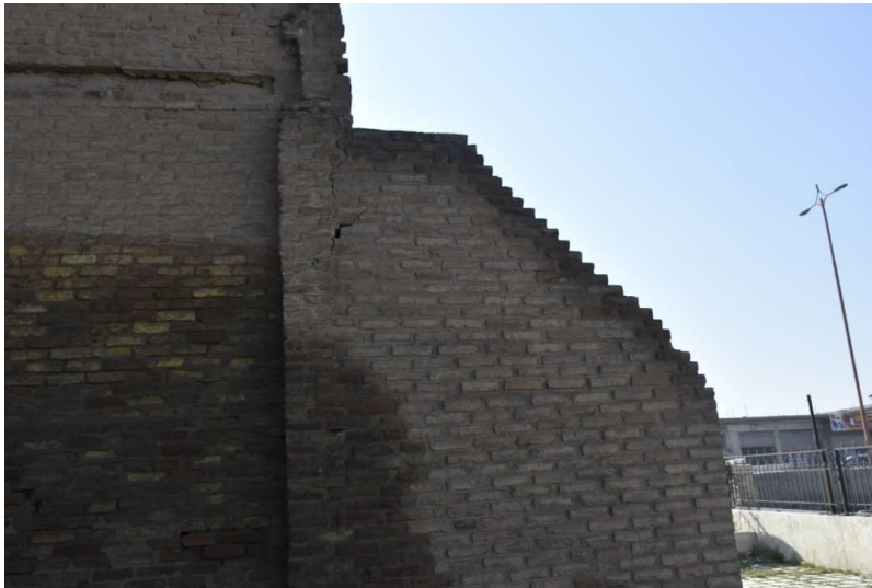
A slight crack in one of the pillars supporting the Baghdad Gate
