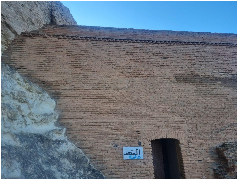
High tower façade, traces of cracks
