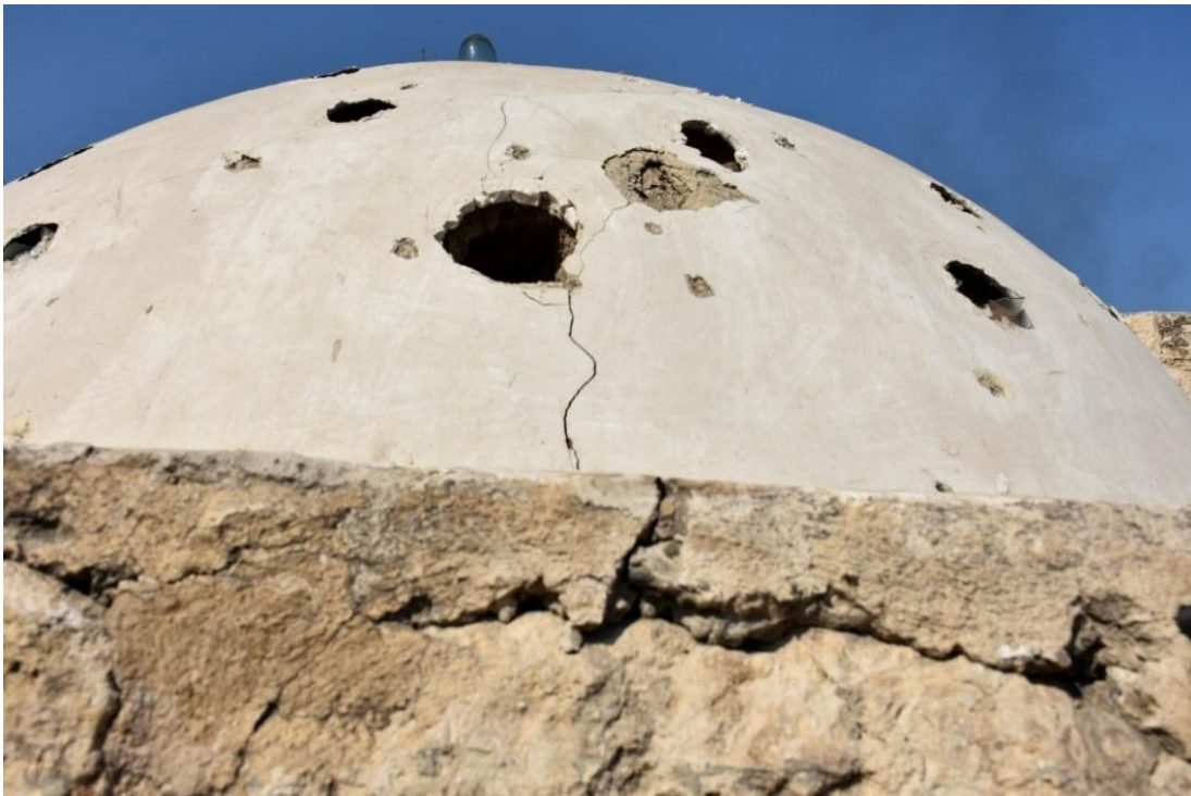
Cracks in one of the domes of the Ottoman bath in Manbij
